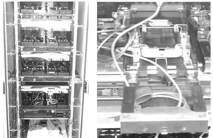
Picture 1: Swisscom Installation. One rack with device pools (left) and one slide-in module for a device (right)
